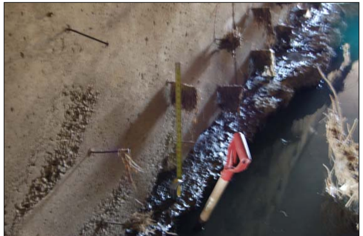
Scour under Foundation
